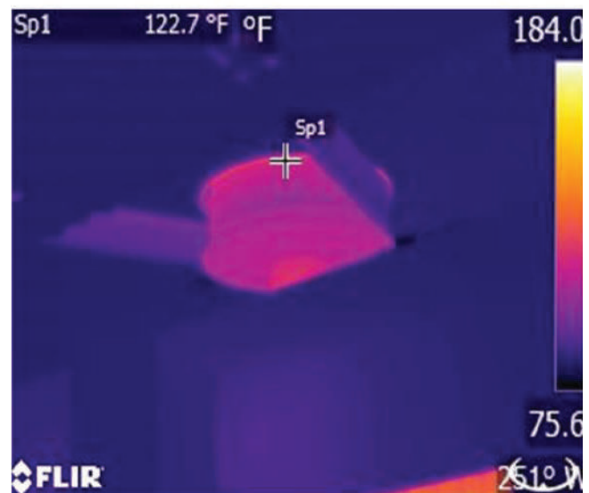
Fin fan pulley thermal profile after implementing the corrective measures
